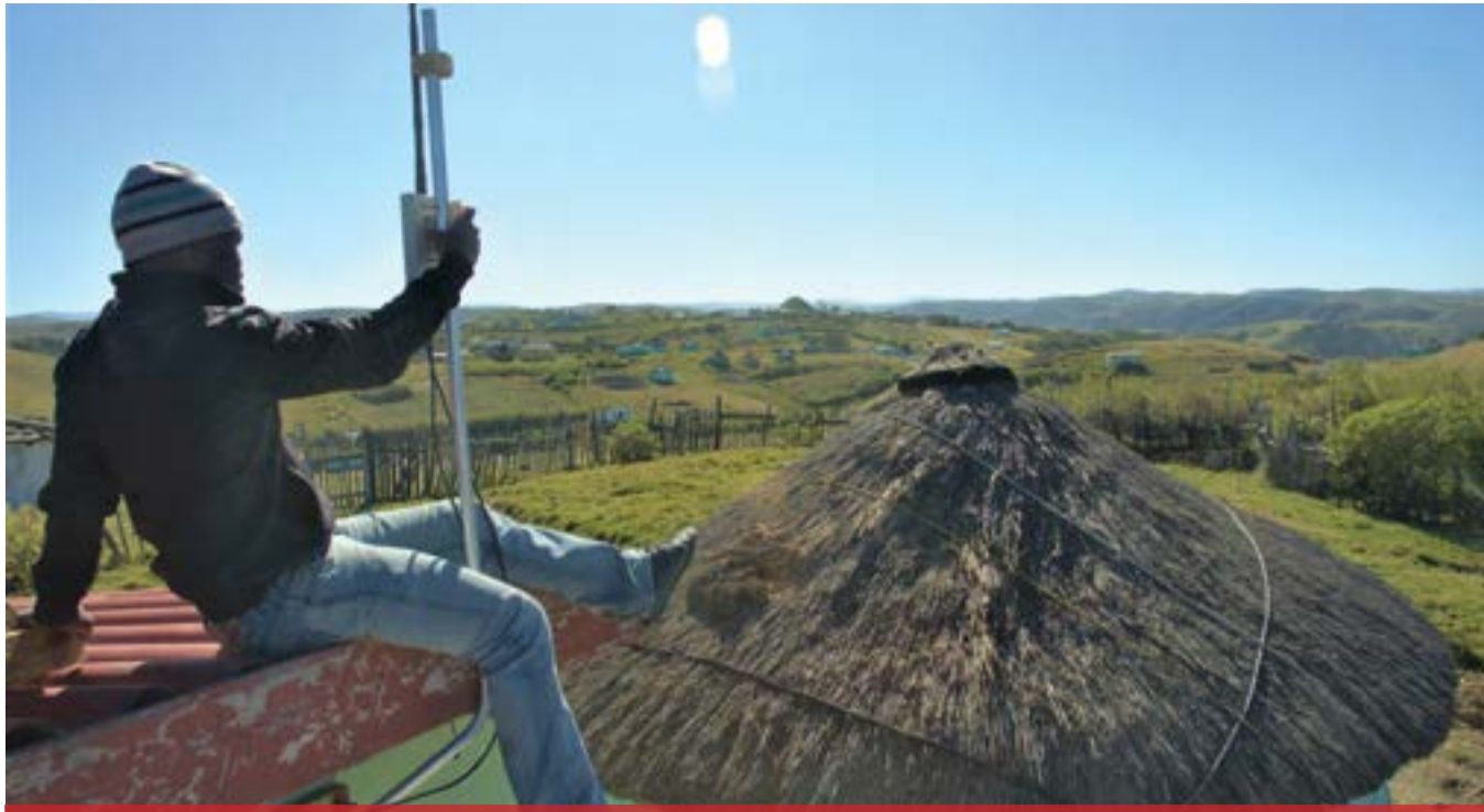
A villager in Mankosi in the Eastern Cape is installing node equipment. Photo: Supplied
